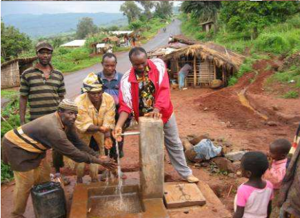
Water flowing out of a completed tap. Field evaluation works by Mr. Yemele Paul. Sarkong community jubilating.
